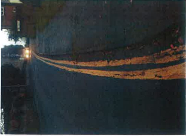
NEPP Officer's Investigation Report from site visit to Mount Pleasant Rd in Saffron Walden
